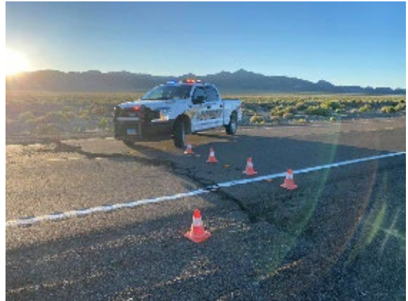
Earthquake in NV Photo Source: The Nevada Independent
