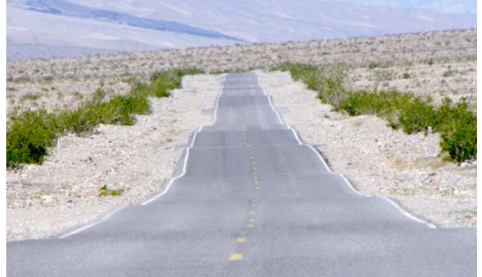
Figure 1. Scotty's Castle Road in the Mojave Desert crossing an alluvial fan, looking northwest. Enhanced creosote growth on the sidecast banks is evident.
